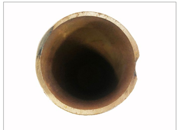
Plate 2: Boiler firetube showing depth of under-deposit corrosion.
