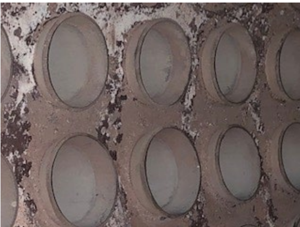
Plate 1: Photograph of mud drum and boiler tubes taken during annual inspection showing the gradual clean-up of the boiler fouling due to use of Visentia V-GUARD internal boiler treatment.
